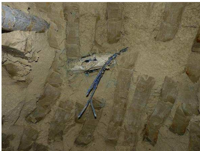
Figure 69: Broken cables during the bentonite removal
