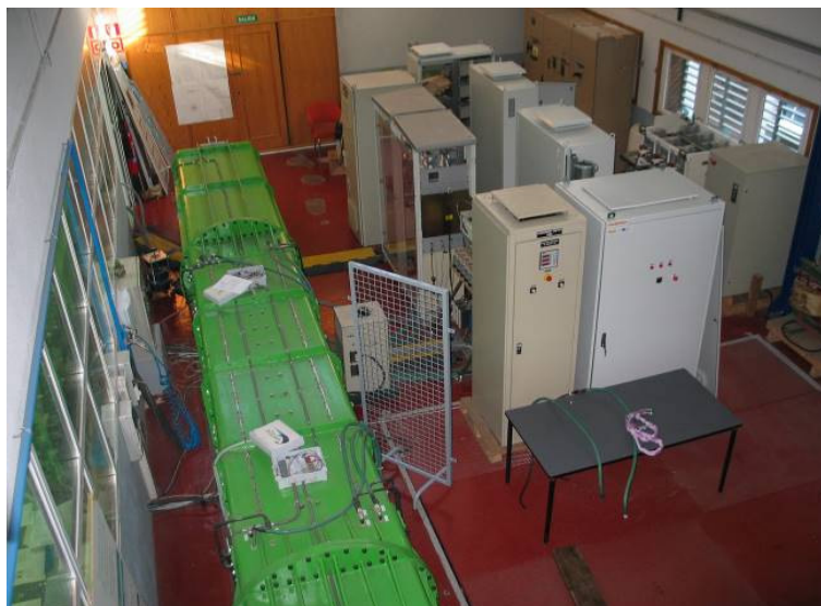
Figure 3. Switched Reluctance Linear Generator during Dry Testing.
