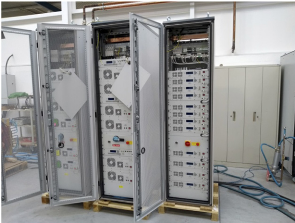
Figure 24. The three cabinets containing the power supplies during the factory tests.
