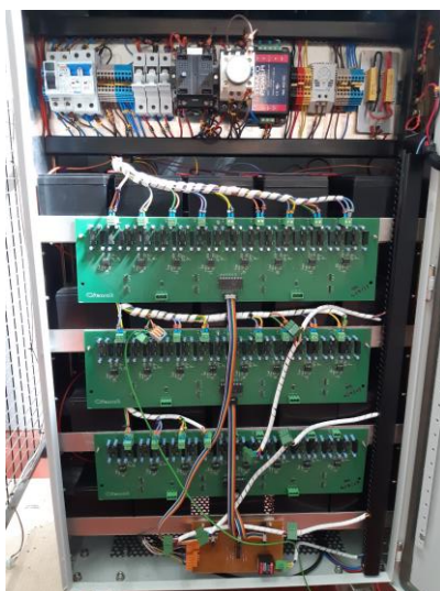
Fig. 15. Battery set for the experiments. 480 V in a string of 40 modules of 12 V per module.
