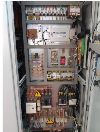
Fig. 17. Power inverter control unit, DSP, and protection systems.
