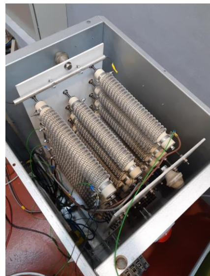
Fig. 18. Three-phase resistive load in terminals of the power inverter.
