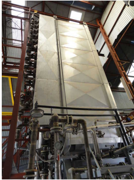
Figure 2: MED plant at PSA
