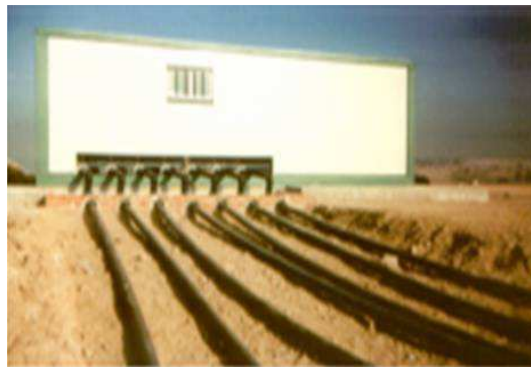
Illustration 13: Regulating and metering station
