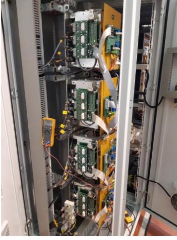
Fig. 11. 140 kW power inverter.
