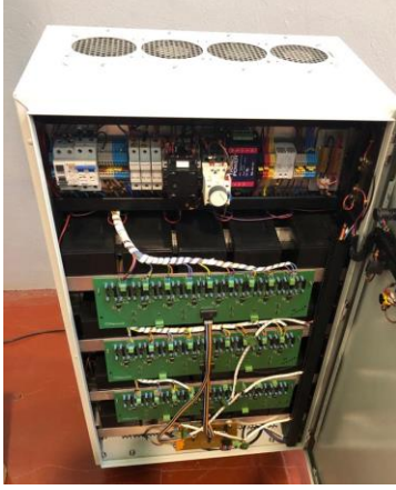
Fig. 13. 480 V Battery pack [1 string of 40 modules of 12 V DC each].
