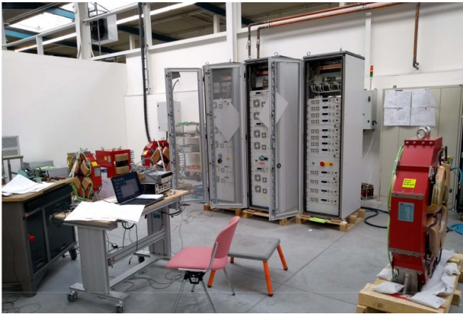
Figure 26. Magnet power supplies during tests at the factory with the real loads.
